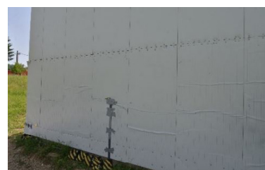
Fig. 2. Blast tests on site: a) structure ready for testing, charge in position; b) the fireball expands; c) deformed shape and damages in the walls
